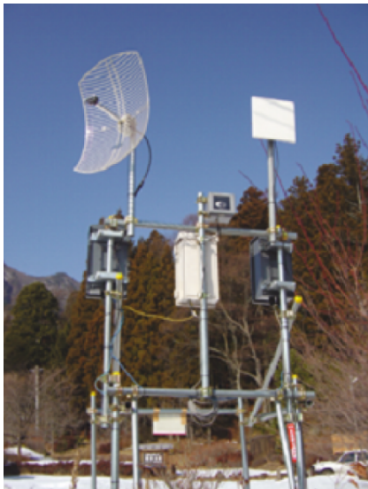
FIGURE 17: Yakushi Park relay station.
