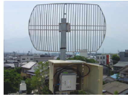
FIGURE 4: An installation example of a parabolic antenna and a wireless LAN unit to a steal pipe.
